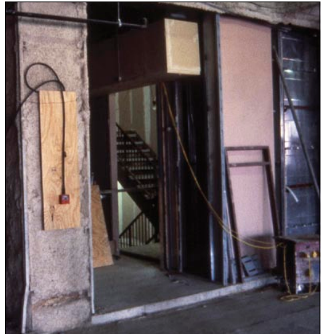
Figure 8(b) This escape route will quickly fill with smoke in a fire because no fire door is fitted
